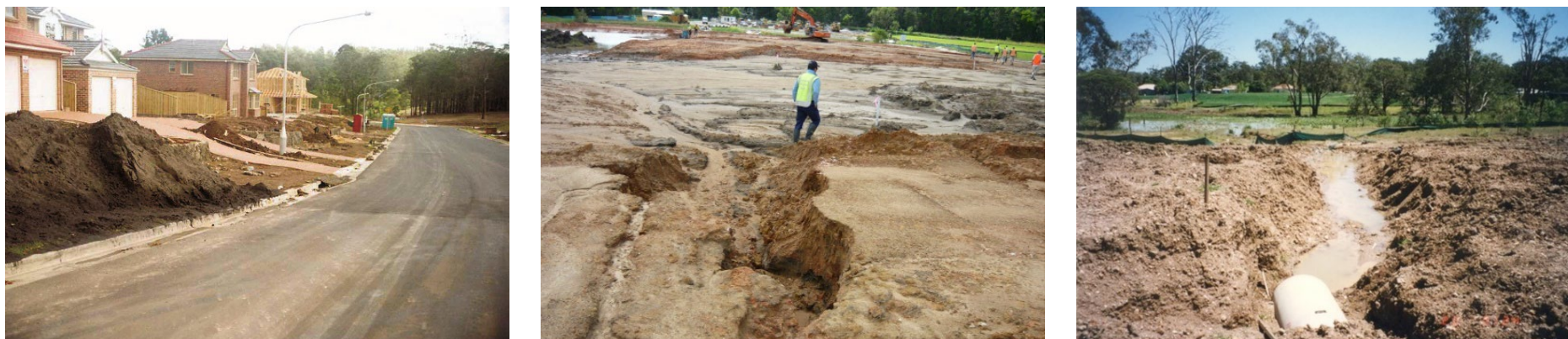
Figure 8. Examples of non-compliant building and development sites.
