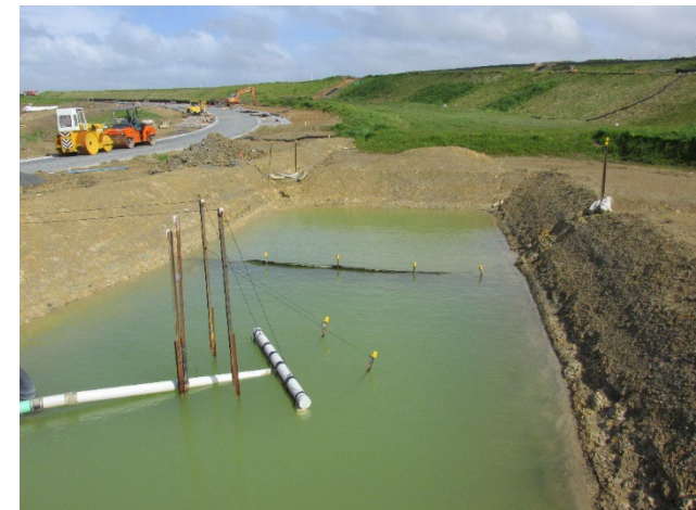
Figure 13. Example of compliant site with a high efficiency sediment basin.
