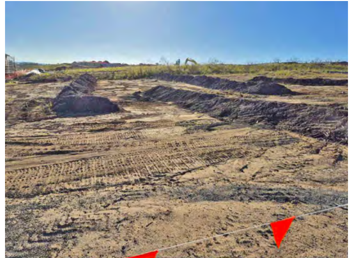
Mulch berm (Source: Topo Group).
