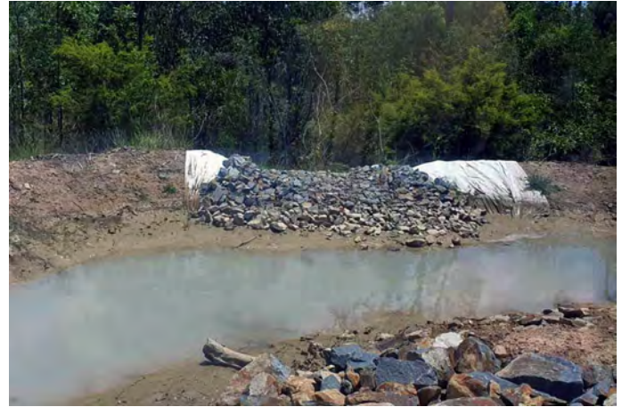
Rock filter dam (Source: Topo Group).
