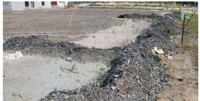
Mulch berm with upslope 'return' being used on a small construction site (Source: Catchments and Creeks).
