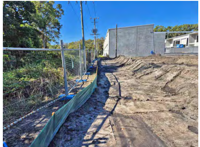
Sediment fence (Source: Topo Group).
