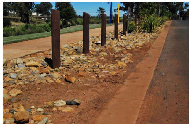
Figure 6 Swale with excessive sediment
