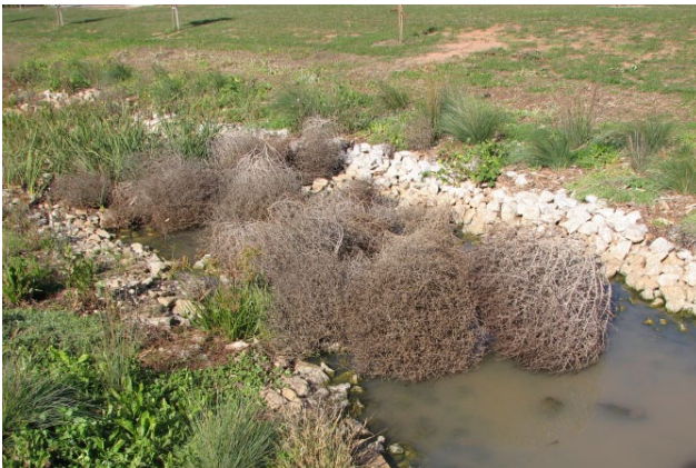
Figure 3 Swale with ponded water due to uneven longitudinal profile and poorly draining soil
