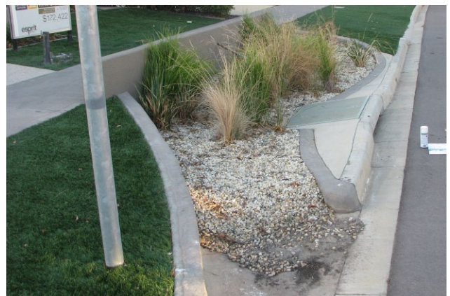
Figure 13 Bioretention system where there is poor distribution of water across the surface because the surface level of the filter media has been incorrectly constructed above the inlet level
