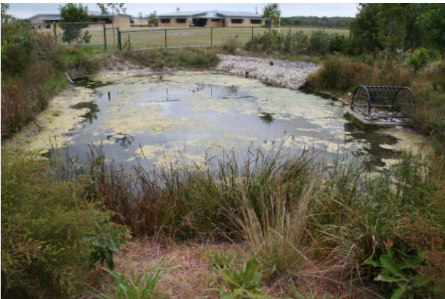
Figure 34 Sediment basin with filamentous algae covering the surface
