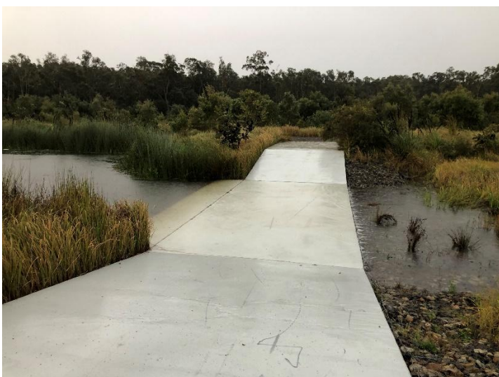
Figure 73. Weir connection from sediment basin to bioretention. Photo credits: Shaun Leinster.
