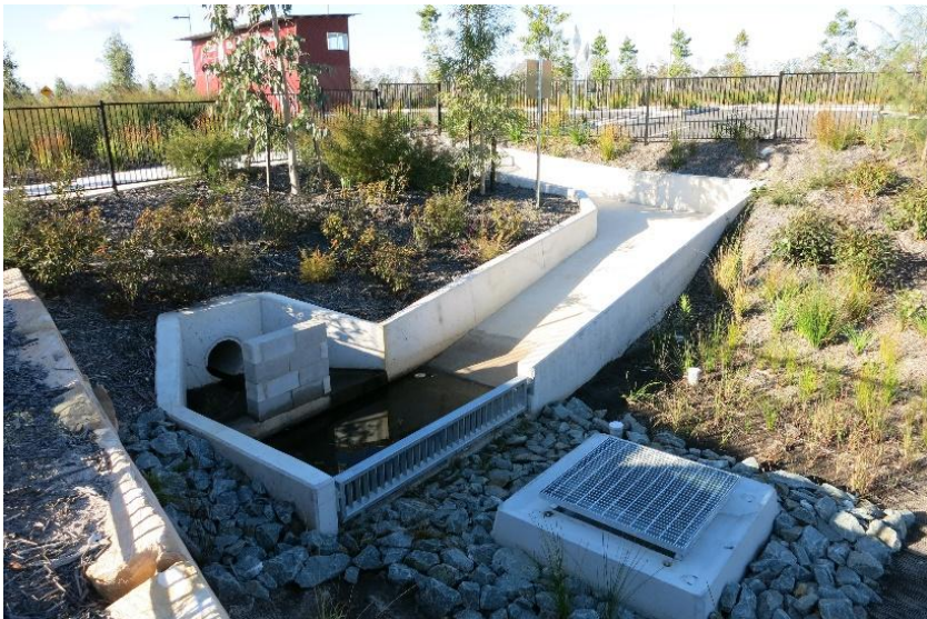
Figure 59. Poorly designed maintenance access. Photo credits: Paul Dubowski.
