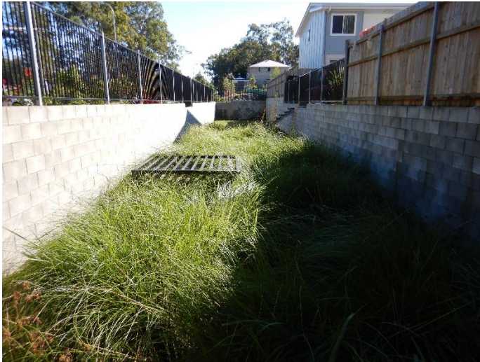
Figure 25. Unacceptable use of walls in a streetscape/on-lot bioretention system. Photo credits: Paul Dubowski.
