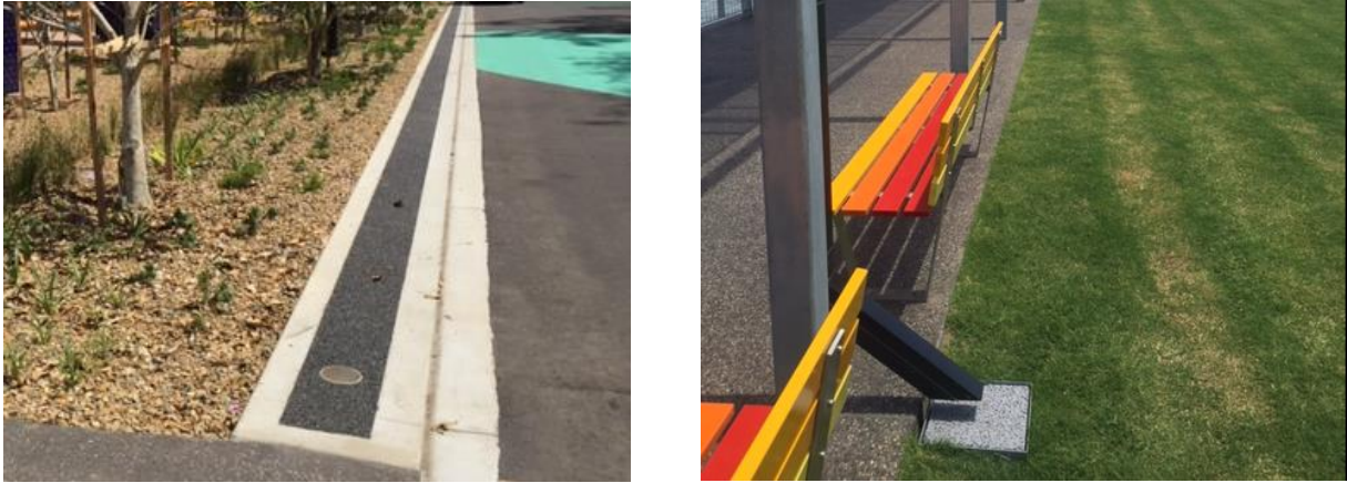
FIGURE 10. PRE-TREATMENT OF SURFACE RUNOFF PRIOR TO DISCHARGE TO WICKING ZONE.
